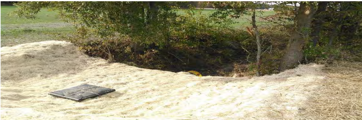
Figure 9. Structure for water control installed in a ditch to help control water level and increase nutrient removal within the ditch.
