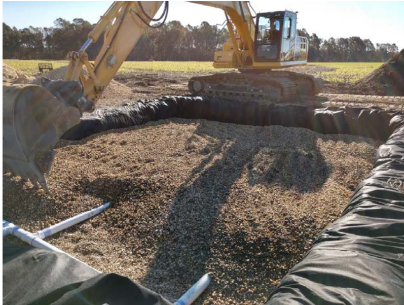
Figure 15. Blind inlet example showing the filter (gravel) being placed over the subsurface perforated drainage pipes.
