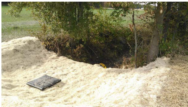
Figure 21. Structure for water control installed in a ditch to help control water level and increase nutrient removal within the ditch.
